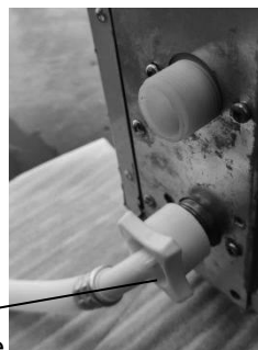
Ice Maker Drainage Pipe
